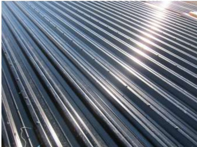
Figure 5.1: Roof-mounted TSC (external view)
