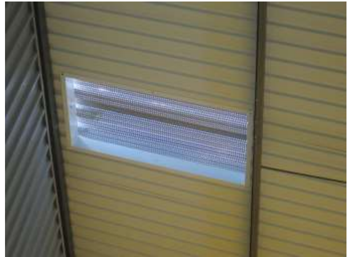
Figure 5.2: Roof-mounted TSC (internal view)
