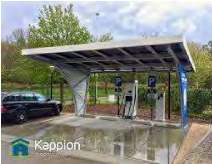
Figure 7.7: Kappion Cantilevered Solar Carport
