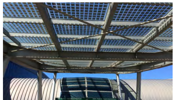
Figure 3.4: Silicon PV in glass entrance canopy
