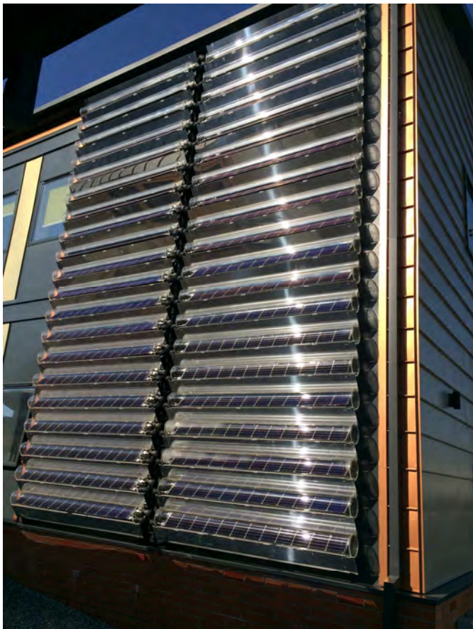
Figure 4.5: PV-T tubes on Active Office
