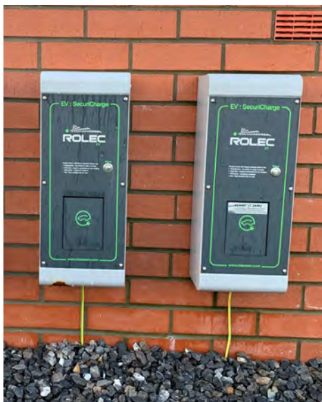
Figure 7.4: Rolec Securicharge wall unit
