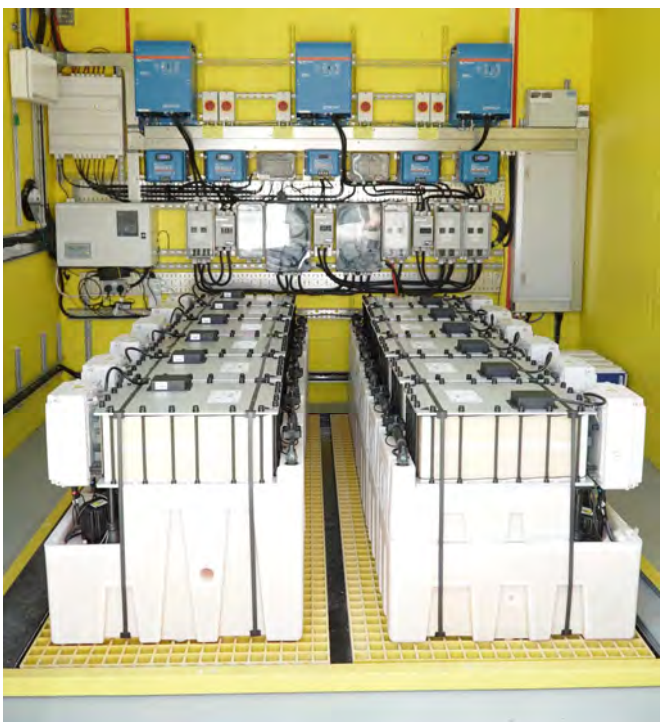
Figure 5.2: Flow batteries in the Active Classroom
