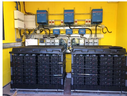
Figure 32: The Aquion batteries inverters and charge controllers
