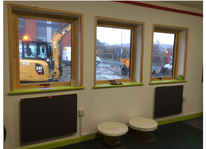
Figure 43: Warmth and Wellbeing Low Temperature Radiant Panel Heaters
