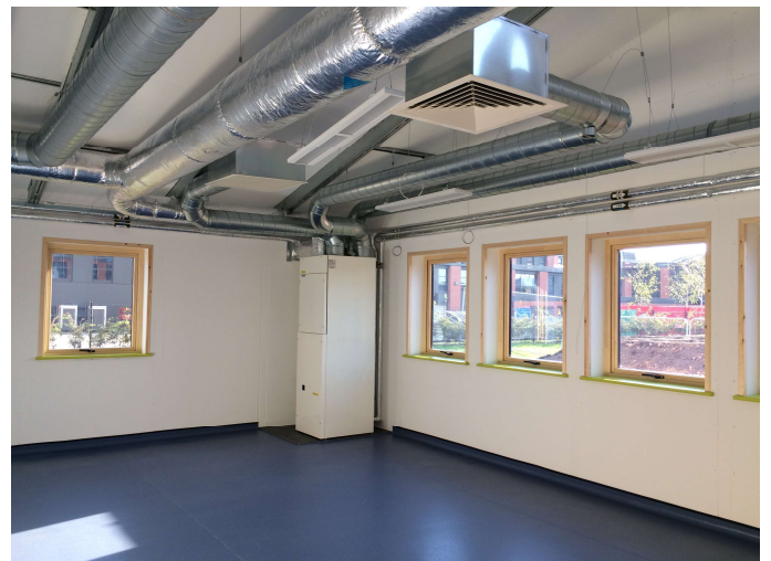
Figure 26: The Genvex unit and air distribution ductwork
